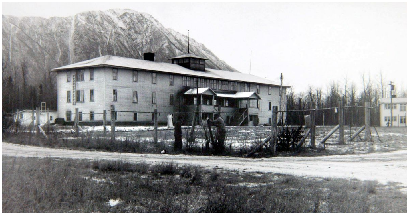
A workman repairs fence at the girl's dormitory at the Eklutna boarding school in this 1938 National Archives photo. (National Archives, File)
